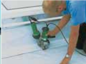
TRIAC DRIVE PID used for welding plastic roofing membranes in a light dome.
